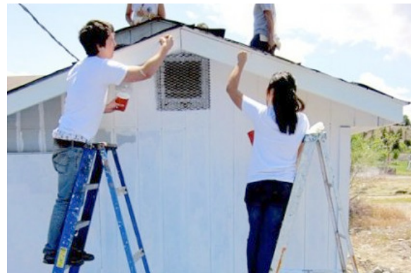
Giving a building a much-needed coat of paint during a Sacred Road mission trip.
